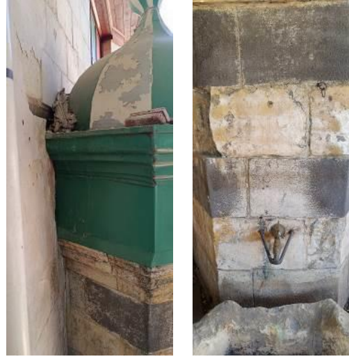
Figure 4. Anthropogenic deteriorations in Kumandan Fountain
