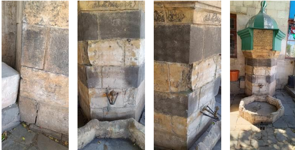
Figure 1. Physical deteriorations in Kumandan Fountain
