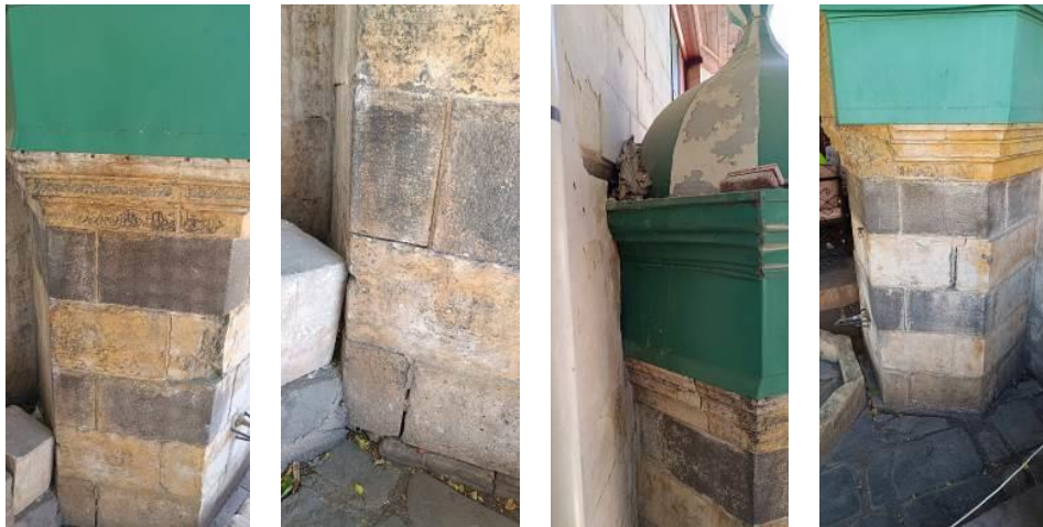
Figure 2. Chemical deteriorations in Kumandan Fountain
