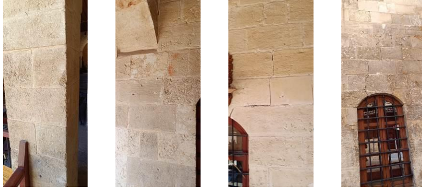
Figure 1. Physical deteriorations in Historical Gümrük Inn
