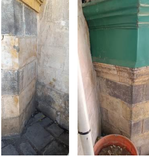
Figure 3. Biological deteriorations in Kumandan Fountain
