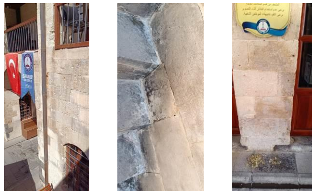
Figure 3. Biological deteriorations in Historical Gümrük Inn
