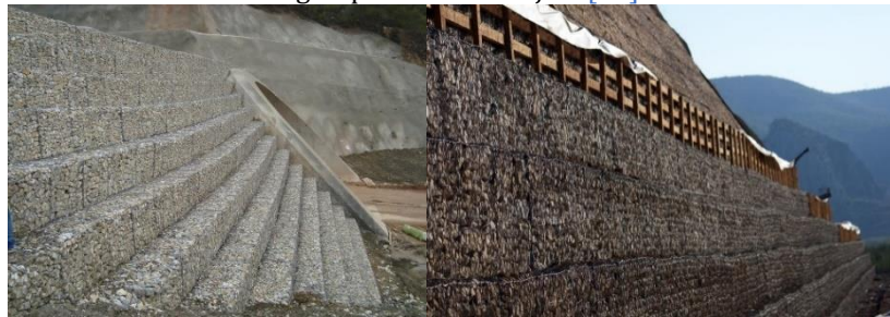
Construction of Terramesh System Retaining Wall within the Scope of Ankara-Istanbul 2nd Stage High-Speed Train Project [17]
