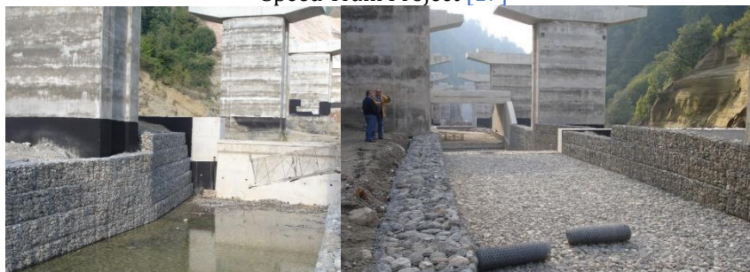
Turkey, Astaldi Bolu Mountain Crossing Stream Bed Improvement Work for the Protection of Viaduct Foundations with Gabion Basket Reno Mattress [18]
