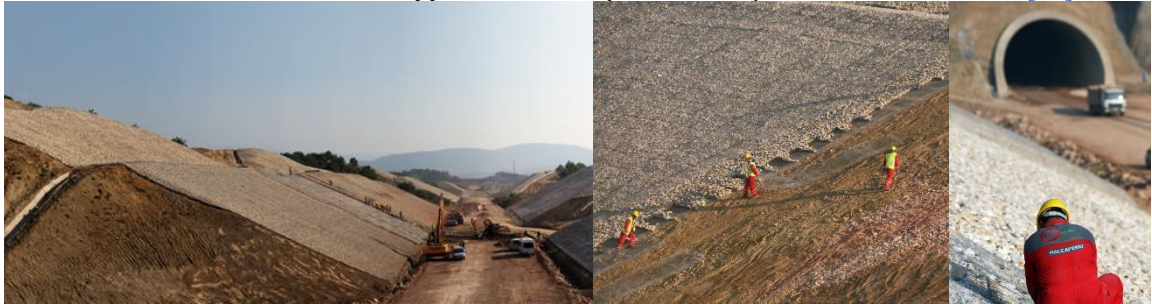
Application of Reno Mattress for Slope Erosion Prevention within the Scope of Ankara-Istanbul 2nd Stage High-Speed Train Project [16]
