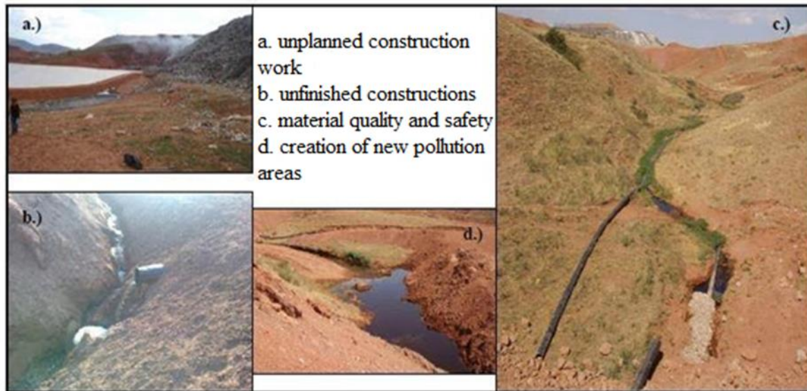
Figure 1. The view of the problems that arise during the construction of a landfill area in pictures a, b, c, d [9]
