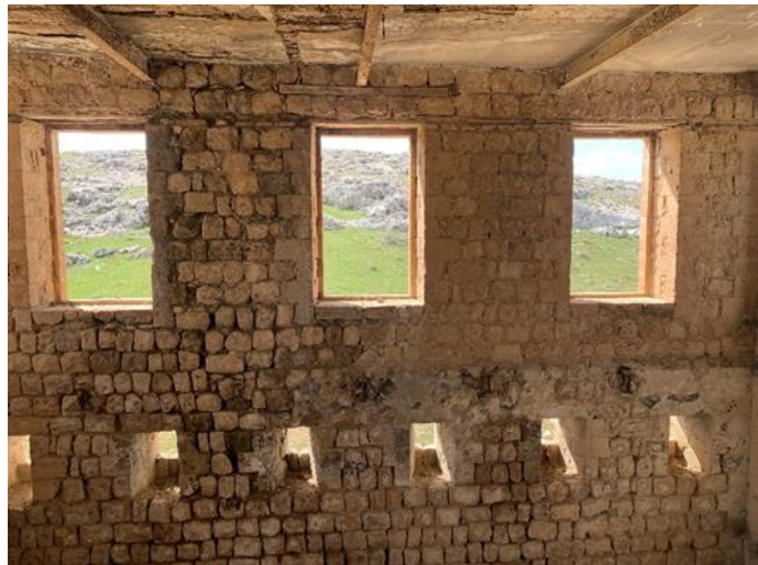
Figure 9. Abrasion of stone material in window cavities
