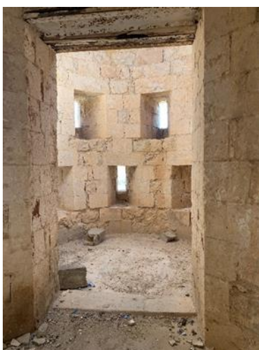
Figure 8. Abrasion of stone material in door openings
