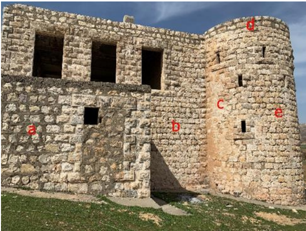
Figure 4. Stone deterioration on the north façade of the building
