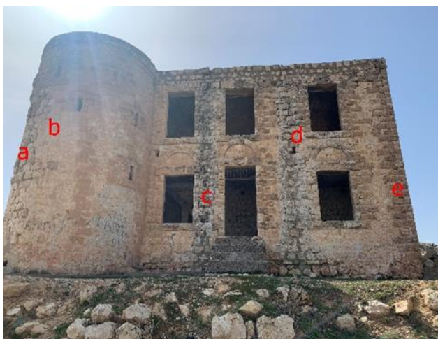
Figure 2. Stone deterioration on the south façade of the building Joint discharge (a), Cement use (b, c), Surface loss (d), Color change (e)
