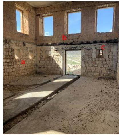
Figure 5. Stone deterioration in the interior of the building
