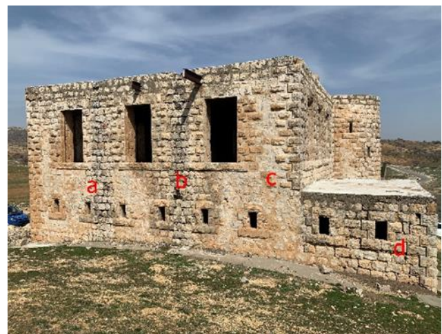
Figure 3. Stone deterioration on the eastern façade of the building Joint discharge (a), Cement use (b, c), Surface loss (d)
