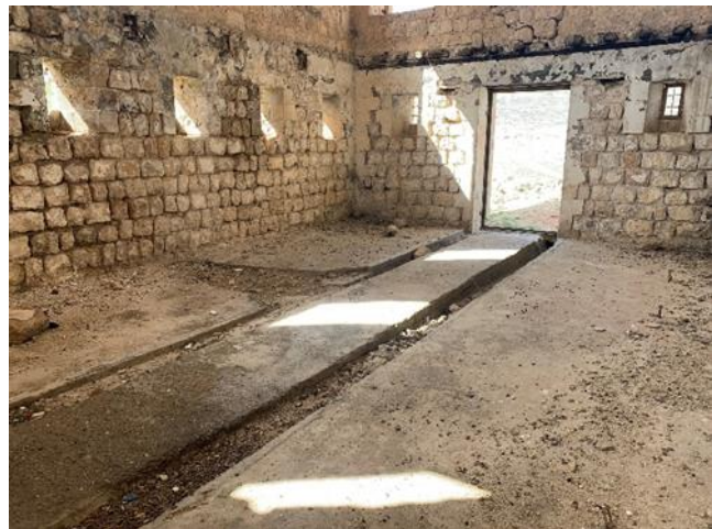
Figure 7. Abrasion on the ground floor layer
