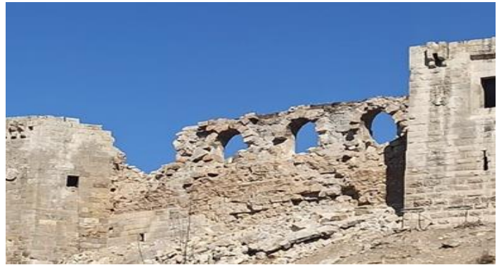
flexural or shear cracks (4a)
