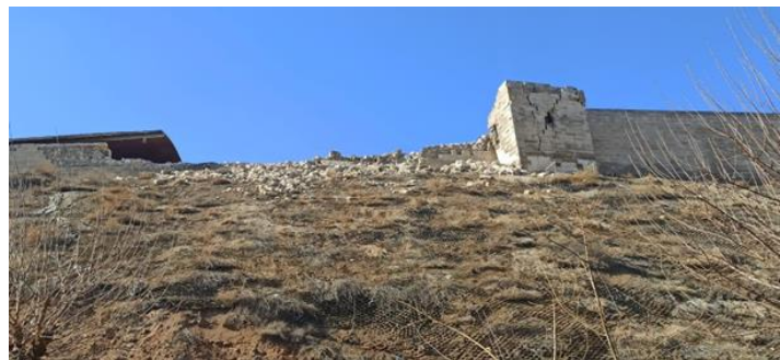
overturning of walls caused by the dynamic thrust of the earth (5b)
