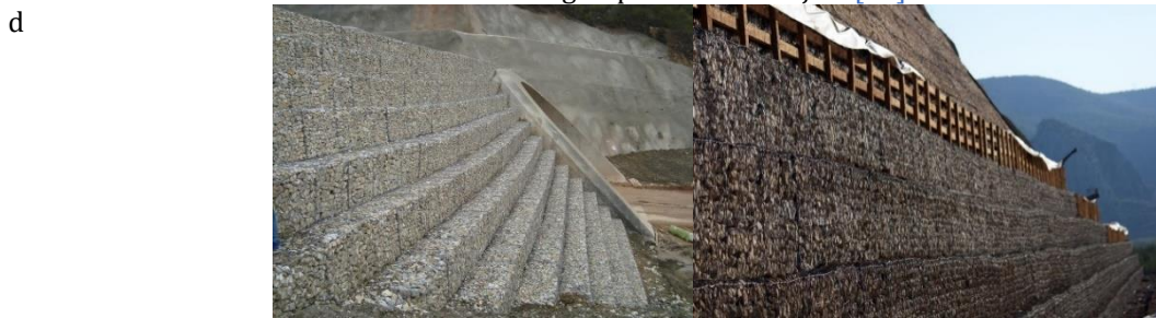
Construction of Terramesh System Retaining Wall within the Scope of Ankara-Istanbul 2nd Stage High-Speed Train Project [17]
