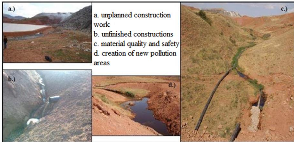
Figure 1. The view of the problems that arise during the construction of a landfill area in pictures a, b, c, d [9]
