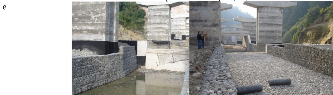
Turkey, Astaldi Bolu Mountain Crossing Stream Bed Improvement Work for the Protection of Viaduct Foundations with Gabion Basket Reno Mattress [18]
