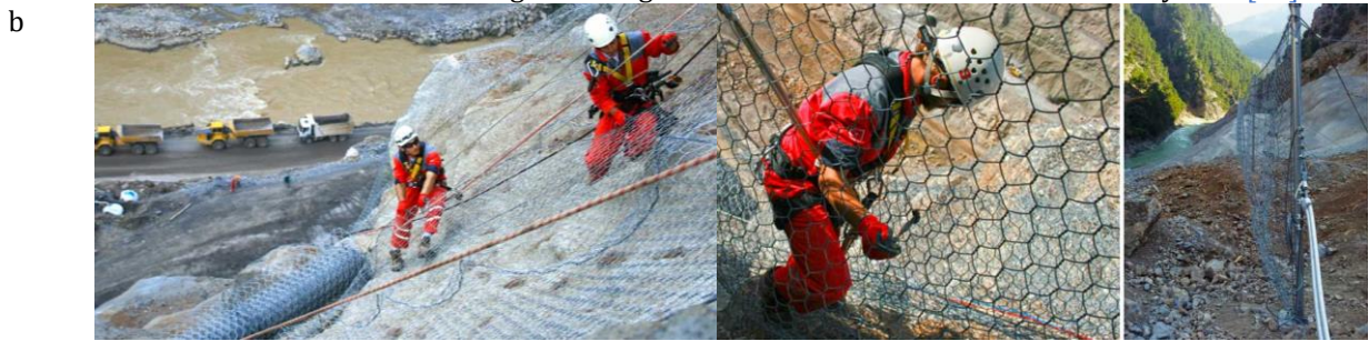
Rock Barrier and Steel Grid Application of Kavşakbendi Project- Gabion Wire Mesh [15]
