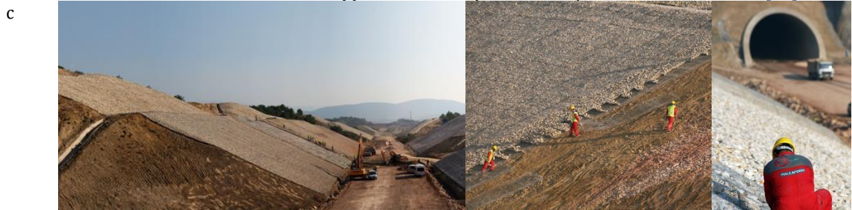
Application of Reno Mattress for Slope Erosion Prevention within the Scope of Ankara-Istanbul 2nd Stage High-Speed Train Project [16]
