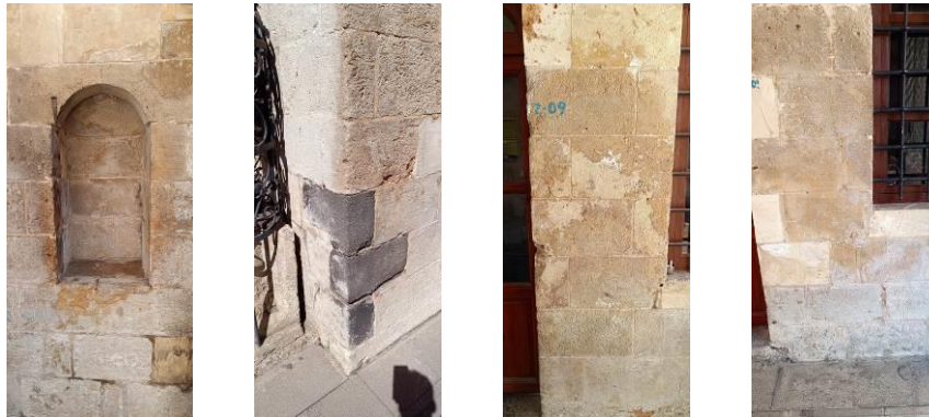
Figure 2. Chemical deteriorations in Historical Gümrük Inn
