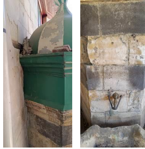
Figure 4. Anthropogenic deteriorations in Kumandan Fountain
