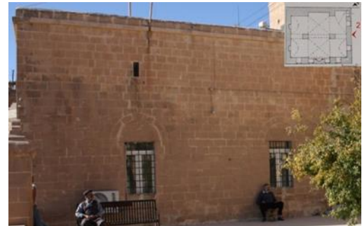
Figure 3. Colour change, use of cement on the wall of façade nr. 2
