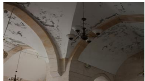
Figure 4. Material loss in the plaster on vaults
