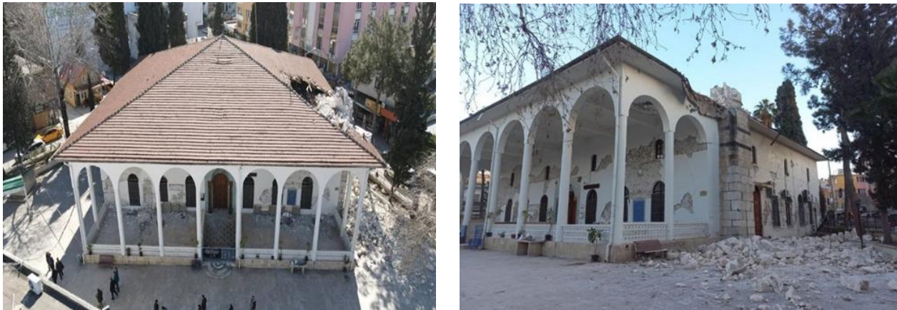
Figure 11. Damage Image After the February 6 Earthquakes [30, 36].
