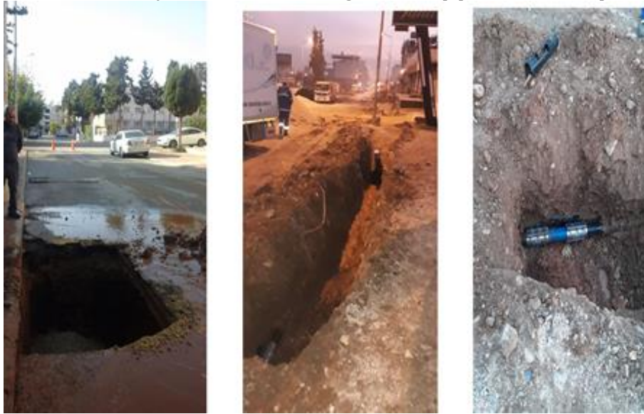
Figure 2. General situation of the pipeline faults
