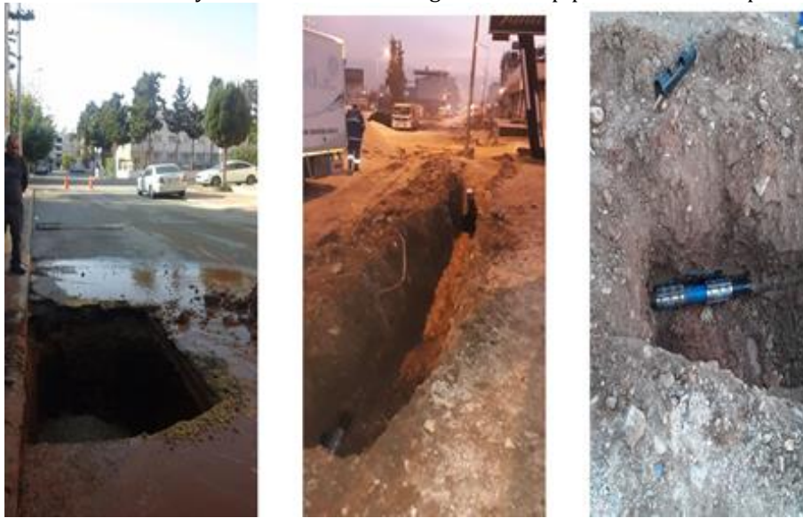
Figure 2. General situation of the pipeline faults
