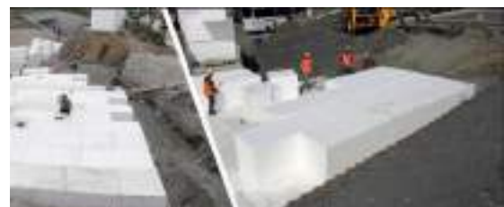
Figure 3. Vibration damping with EPS on the infrastructure instead of a conventional compressed earth fill.
