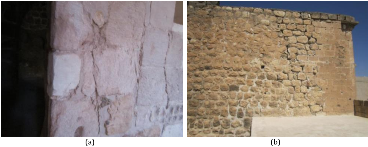
Figure 6a. General view of static problems on the interior wall of the house Figure 6b. General view of static problems on the wall of the neighboring house
