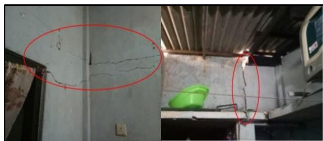
Figure 5. Wall Cracks in Damaged Houses.
