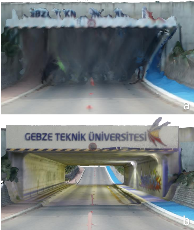
Figure 5. 3D model of the underground pass produced using RGB UAV dense cloud (a) and using the fusion of RGB UAV dense cloud and colored terrestrial laser scanner dense cloud (b)
