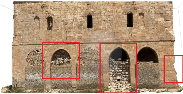
Figure 5. The deformed parts of the historical church
