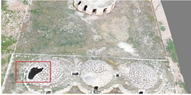
Figure 4. The deformed parts of the historical church
