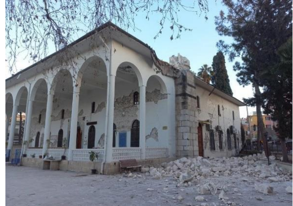
Figure 6: Damage Image After the February 6 Earthquakes (URL_8)
