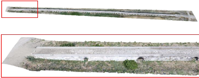
Figure 1. 3D model of the bridge under study. The entire 3D model of the bridge (top), the part of the bridge studied in detail (bottom).
