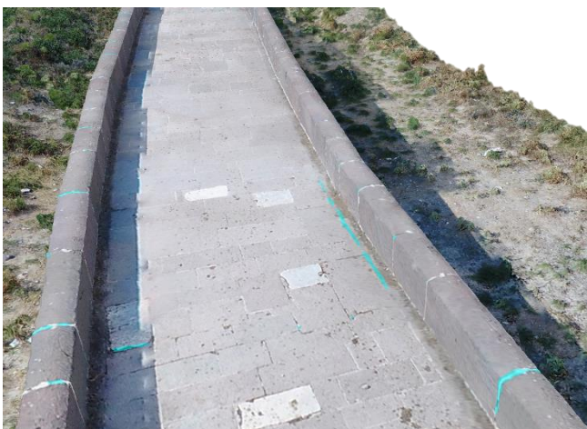
Figure 3. Detected cracks (north view)
