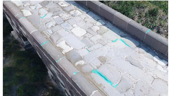
Figure 5. Detected cracks (east view)
