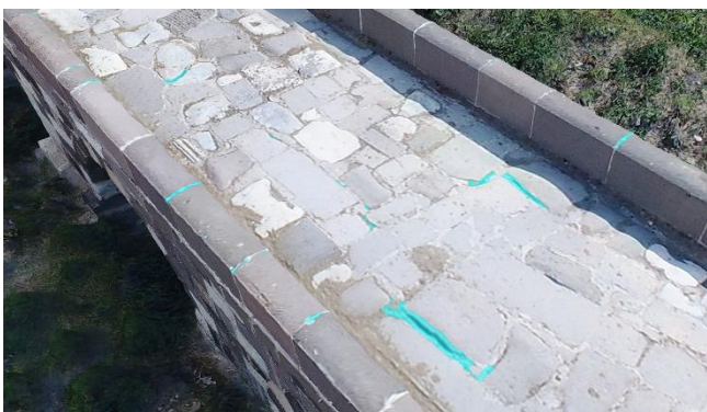
Figure 4. Detected cracks (south view)
