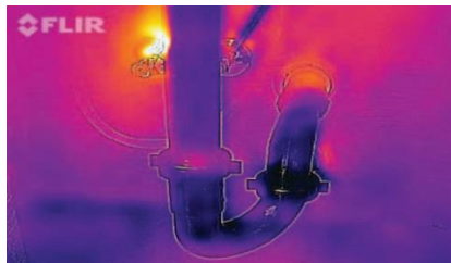
Figure 29. Gas leak detection using a thermal camera [70].
