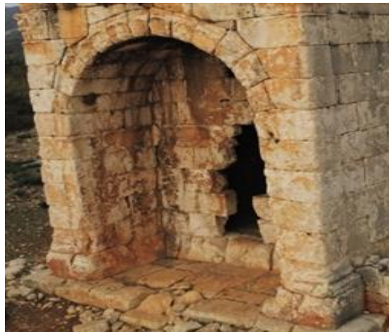
Figure 3. Scaling and discoloration of the feet
