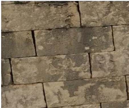
(a) Joint Discharge
