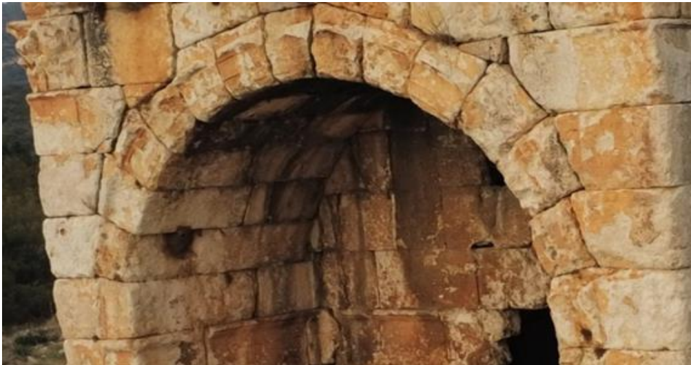
Figure 9. Joint discharge and discoloration in the arch
